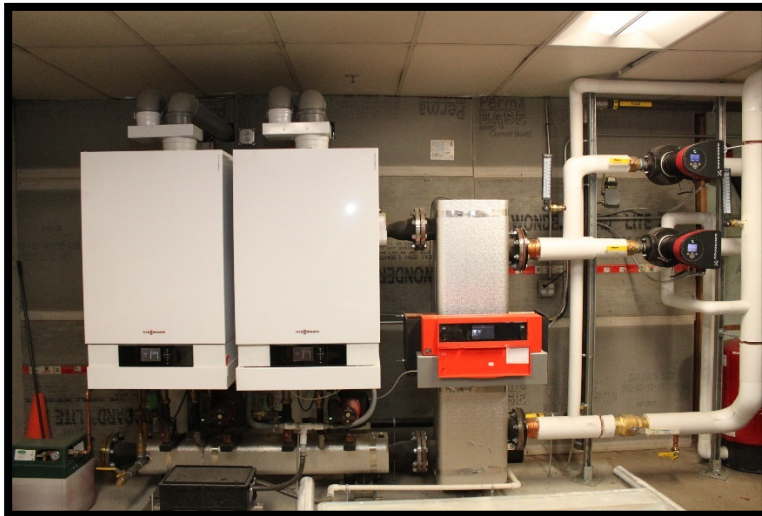
Viessmann, 96% efficiency boilers installed in 2015
